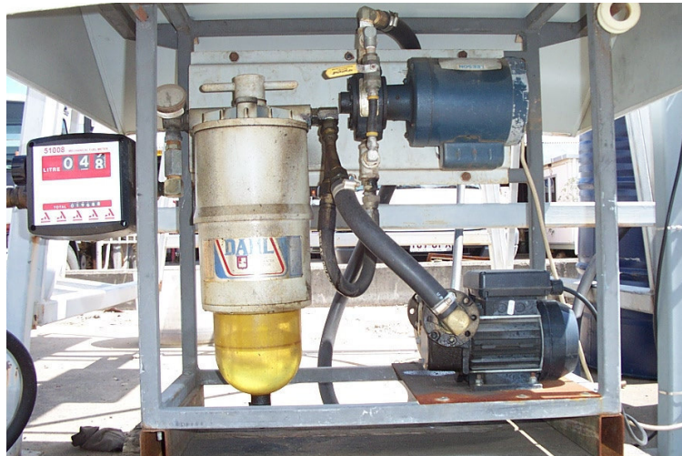
Biodiesel dispensing facility
